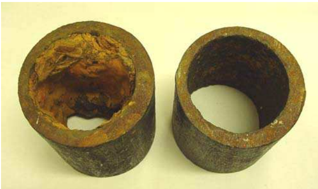
Fig. 9. Example of effective cleaning of a water pipeline after 50 years of use
