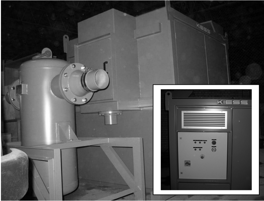
Fig. 19. General view of Vacuum Extractor aggregate type DV 3001 D KIESS including cyclone pollutants separator
