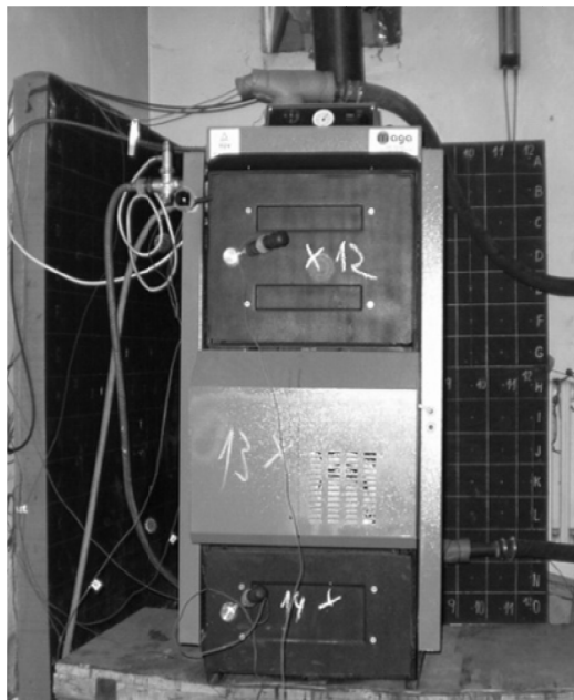
Fig. 1. The hot water boiler MA 23 – test probe connection [14]
