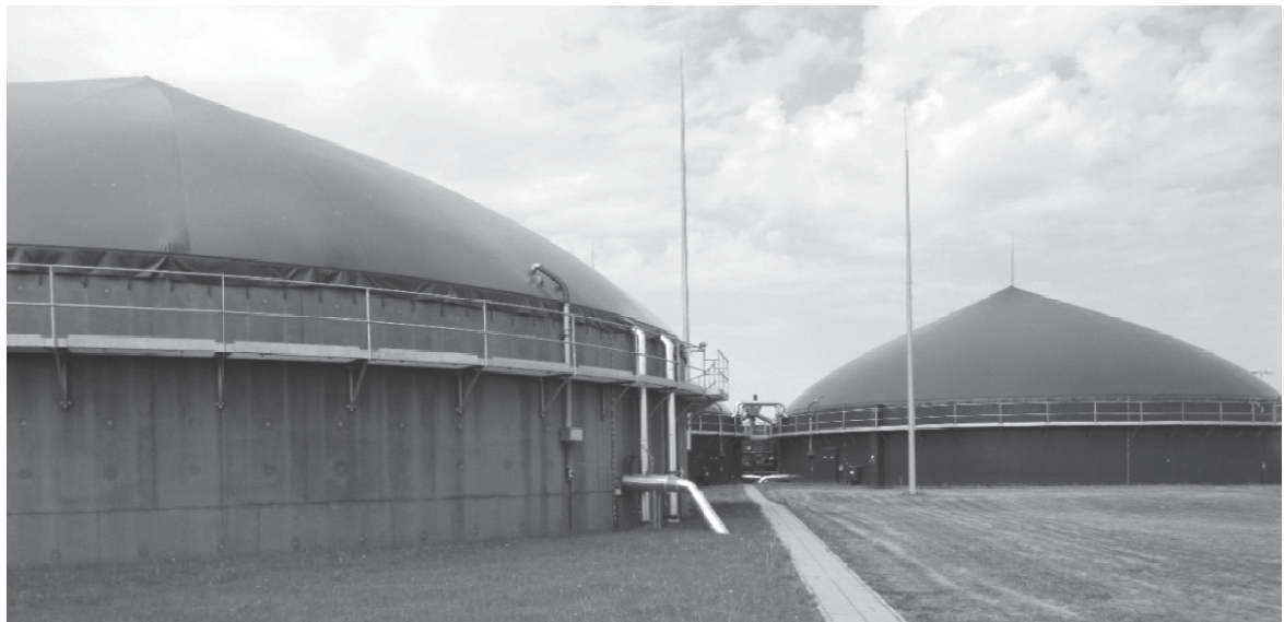
Fig. 2. The storage tank and fermentation chamber located in the Ryboly Biogas Plant
