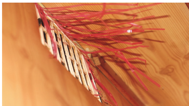
Fig. 4. Backward flow of ventilation air from the ventilation sheet in the bathroom on the ground floor
