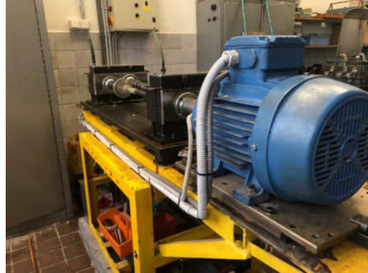
Fig. 2. Three-phase electric motor of Niemann M01
